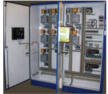
Multi Drive System with Data Acquisition
