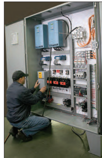
Slitting Line Control
