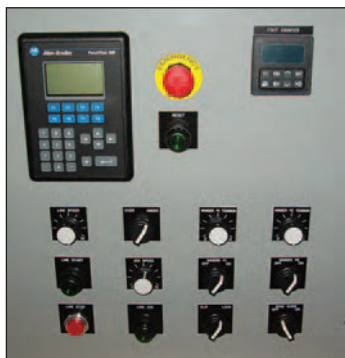
Operator Control Station
