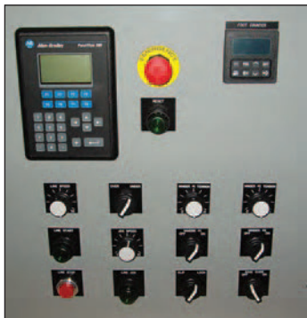
Operator Control Station
